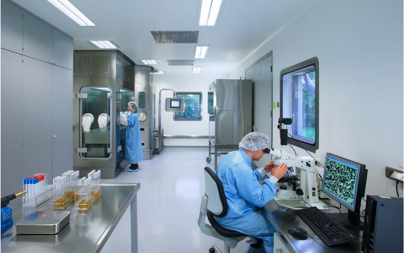
▲ Cleanroom class D with integrated isolator system
